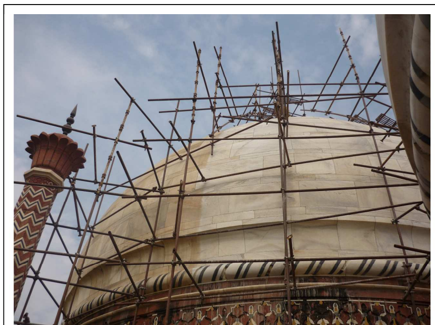
FIGURE 1. A clean surface and an area being prepared for cleaning on a marble Mosque dome at the Taj Mahal
